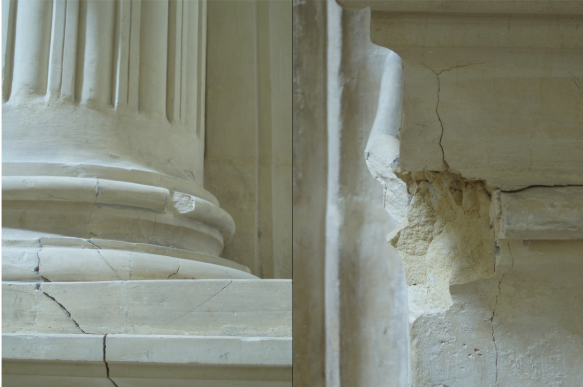
Figure 4 - Some of the observed cracks within the church
